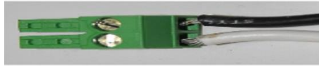
Correct wiring for 2-pin CT plug
